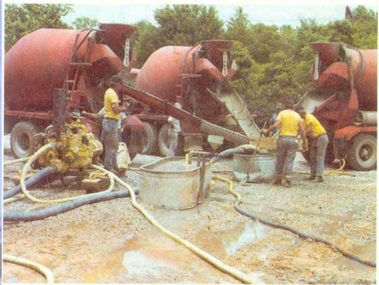
Figure 4.3 Three cement trucks are required to provide enough cement to grout the casing in this 150 m borehole. The cement is pumped from the stock tank into the borehole by a positive displacement duplex pump, shown on the left.
